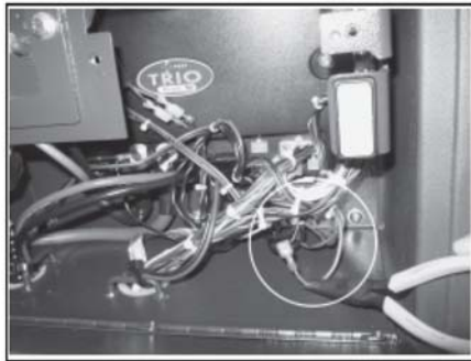
Figure 1 Jumper wire disconnected
